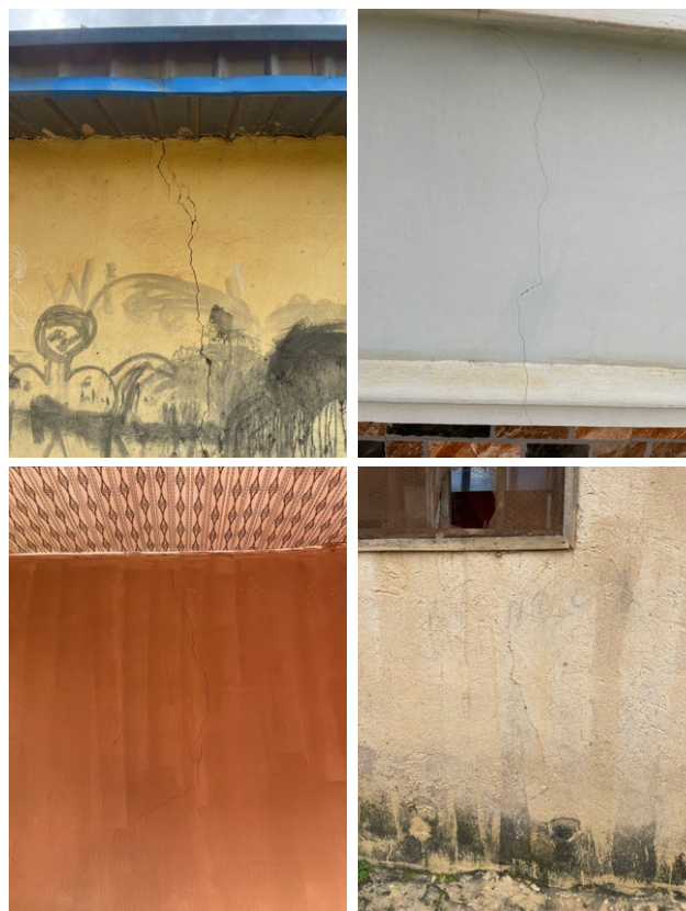
Blasting operations allegedly cause buildings to crack.
